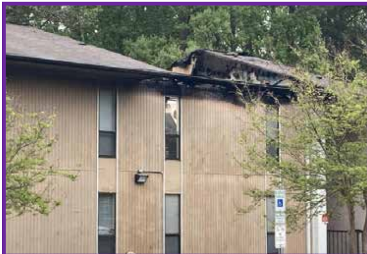
The fire damaged a number of apartments.
